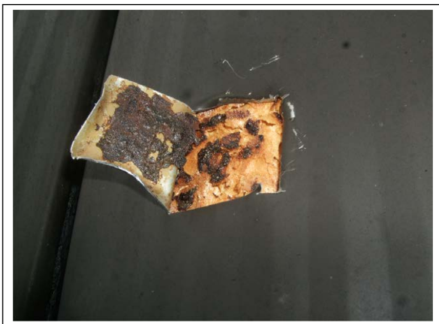
Figure 6 – PIR core material at location exhibiting delamination but where panel coating is still intact
