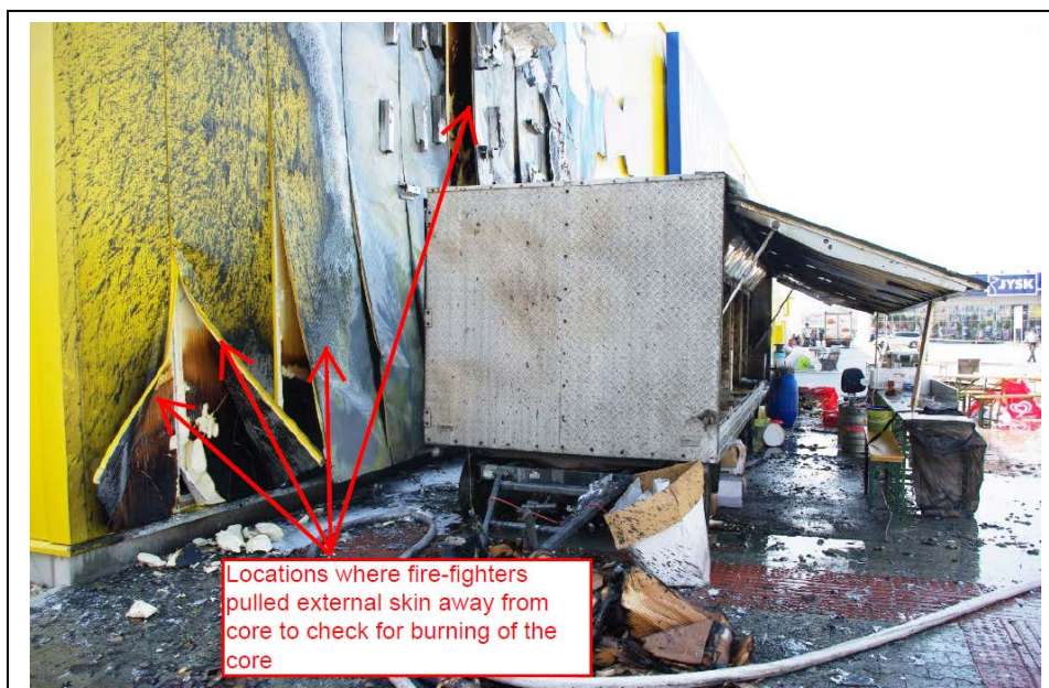
Figure 3 – Points where fire-fighters pulled external skin away from IPN core to check for burning within the core
