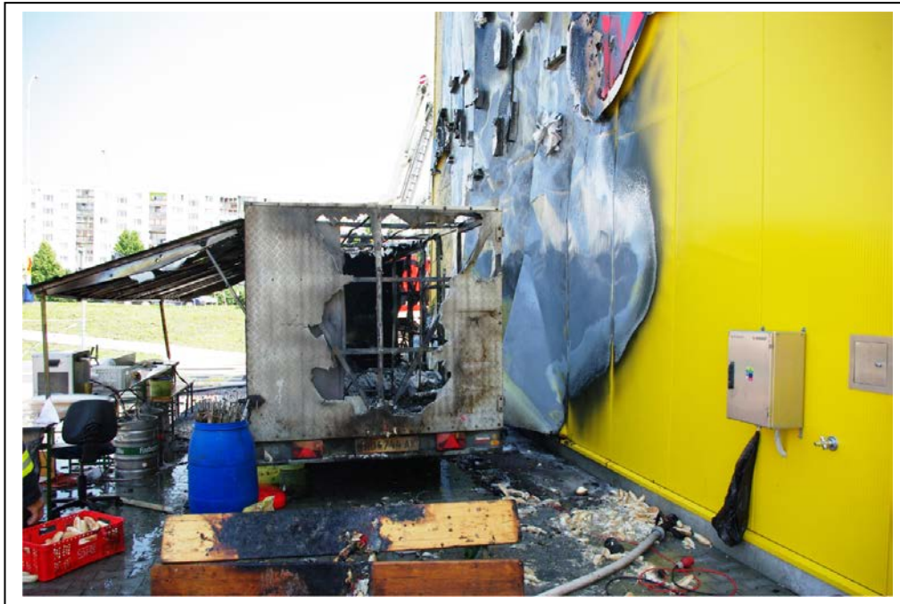
Figure 5 – View of fire damaged grill showing proximity to the building facade
