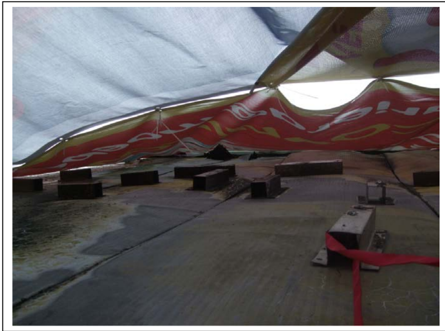
Figure 8 – Close up of surface of panels in area where sign and panel coating have been burned away (the top hat sections are the fixing brackets for the sign)
