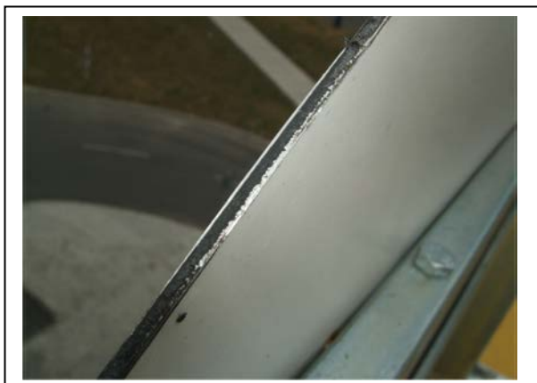
Figure 6 – Top edge of the store's mascot sign showing aluminium composite panel construction
