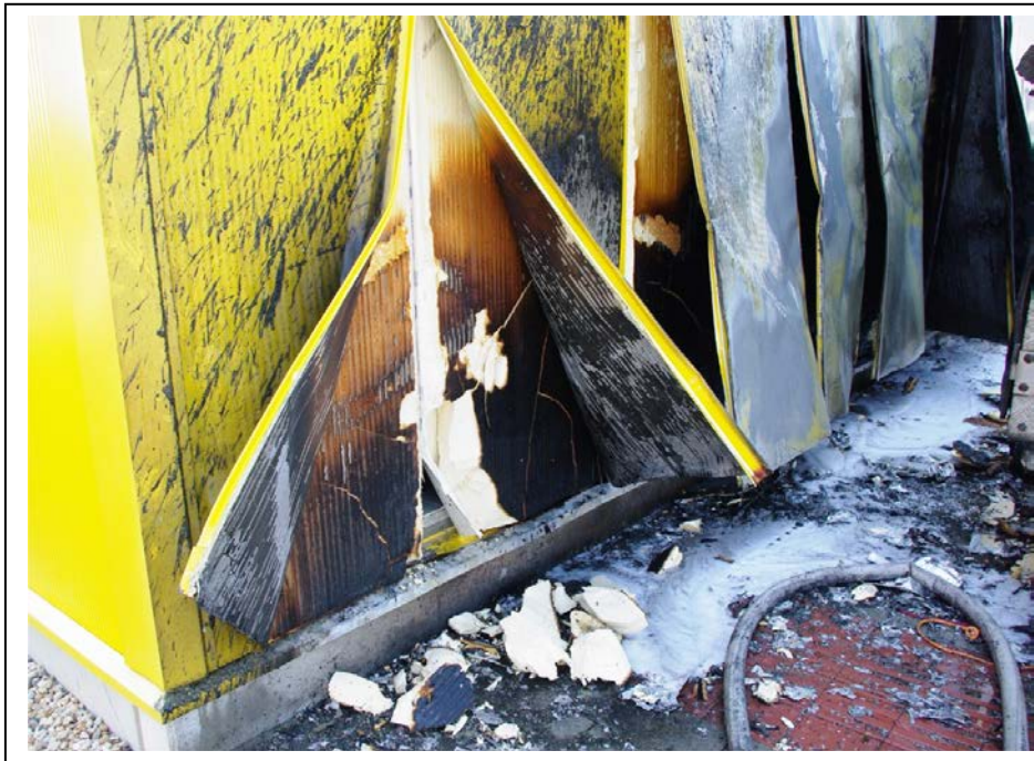
Figure 12 – External steel skin of IPN panel pulled back to show unaffected IPN core material outside area of direct fire plume impingement
