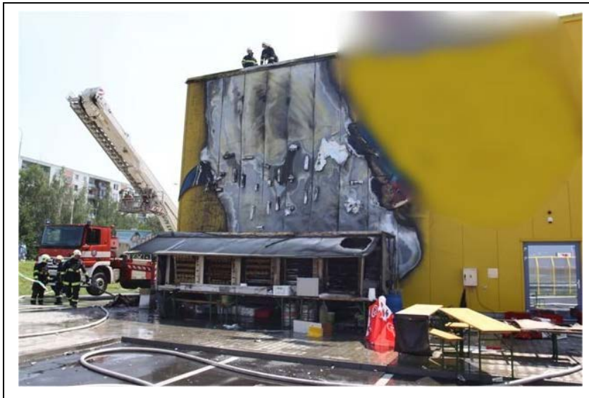
Figure 2 – Photograph of the external wall of the building after the fire showing extent of fire impact on the external façade and the grill in the foreground.
